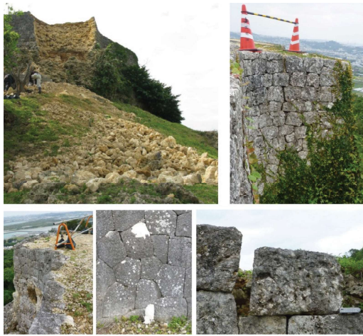
Figure 2. Damage induced by 2010 Off-Okinawa earthquake on Katsuren Castle.
